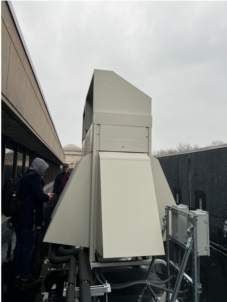
3. Rooftop compressor for the VRF unit
